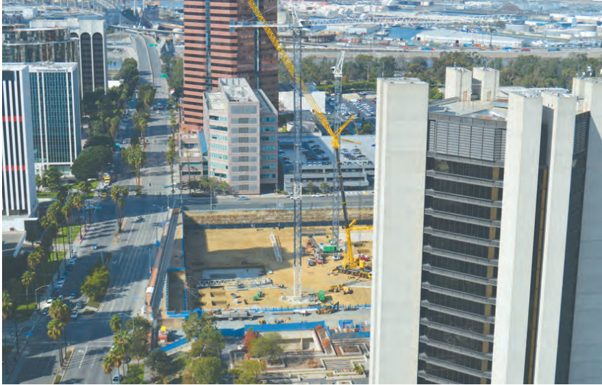
Just past the existing Long Beach City Hall tower, construction has begun on the new Long Beach Civic Center, which will include a new city hall, main library branch and port headquarters, plus multi-family residences, retail and possibly a hotel. (Photograph by the Business Journal's Larry Duncan)
